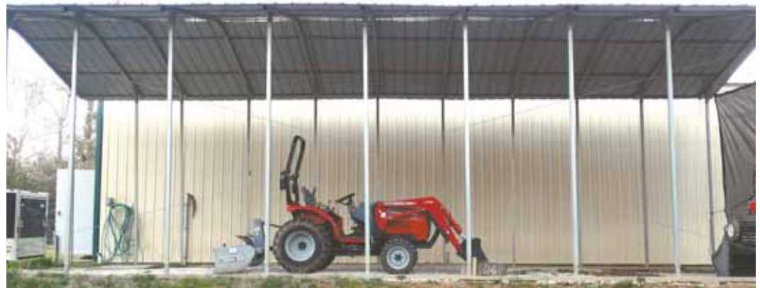
Phil McIntyre used his 50 hp loader tractor and bush hog mower to move this 18 by 40-ft. carport. Chains and pipes were used to stabilize carport's side rails. Then, with chains draped over loader and bush hog, he raised carport off the ground and backed up with the structure around him.
